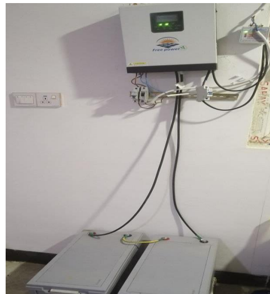
Figure 2: Full Solar system showing the inverter device and the batteries
