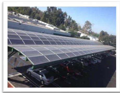
Fig. 9: Picture of the Hybrid station system.
